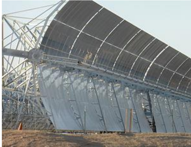
Parabolic trough at a plant near Harper Lake, California fig (1)
